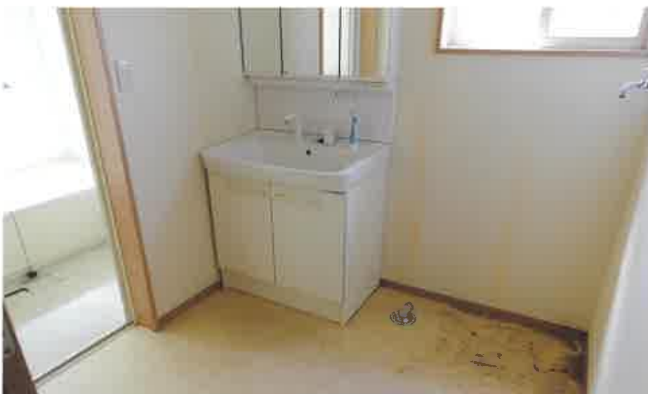
6 (物件2 1階洗面脱衣室)
