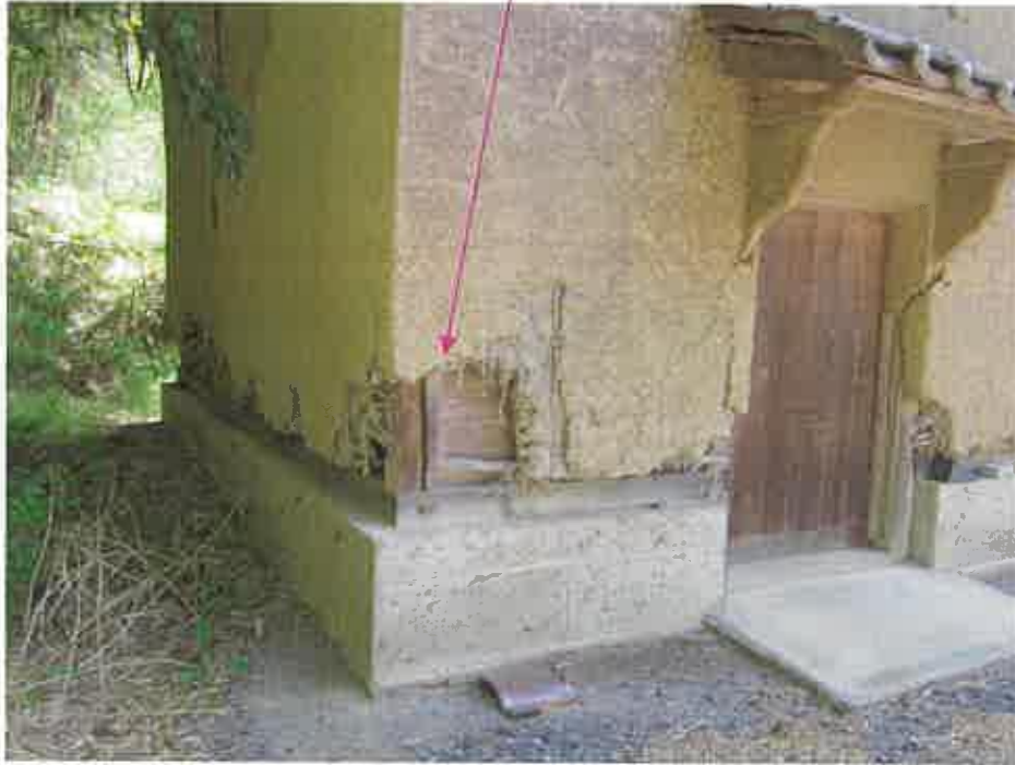
物件3: 物置の外壁の破損
