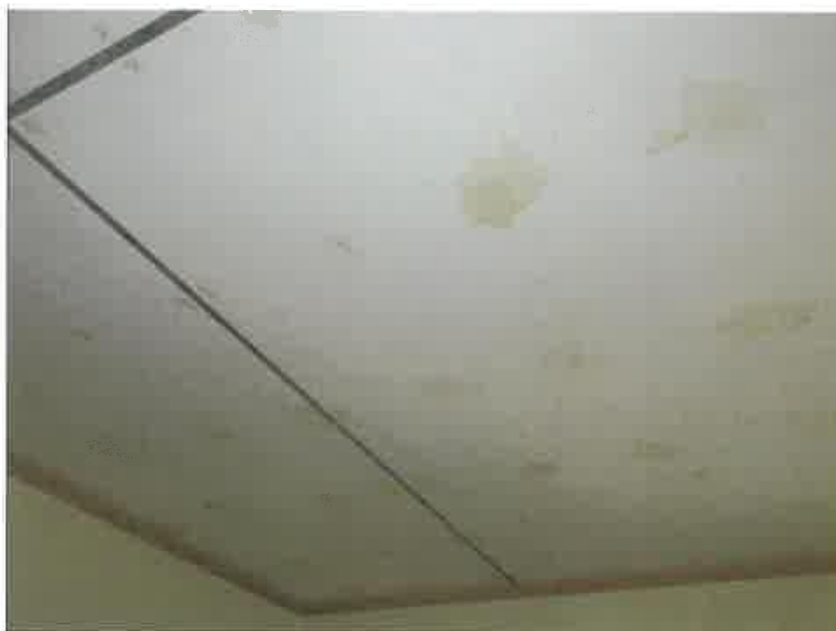
物件2:1階洋室の天井の染み
